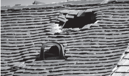
DAMAGE (P. 27, Act. 2)
